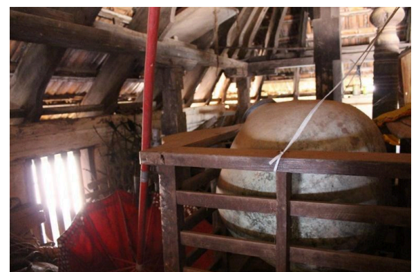
Figure 14. Condition of timber rafters, Thiruvappu. Image: Gopika Jayasree (taken in 2016)
