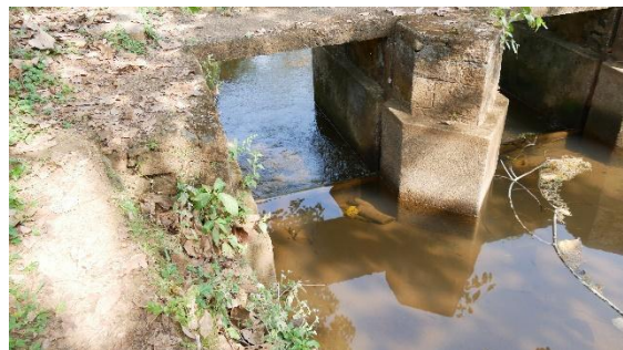
Figure 11. The main canal has slots between the pillars to place planks. The planks would act as a check dam when water has to be diverted to the paddy fields towards the side. Image: JANAL Archives, 2024.
