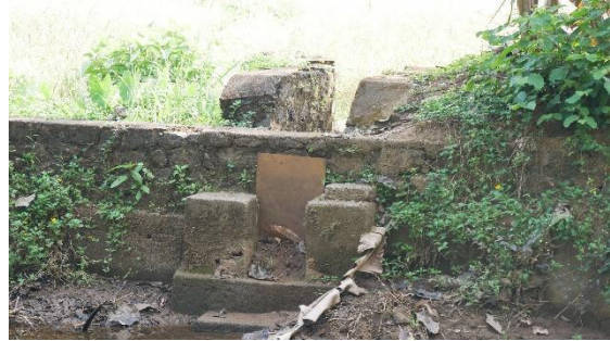
Figure 10. Opening to a varalli from a bigger canal. The opening is closed with a tile at present. Image: JANAL Archives, 2024.
