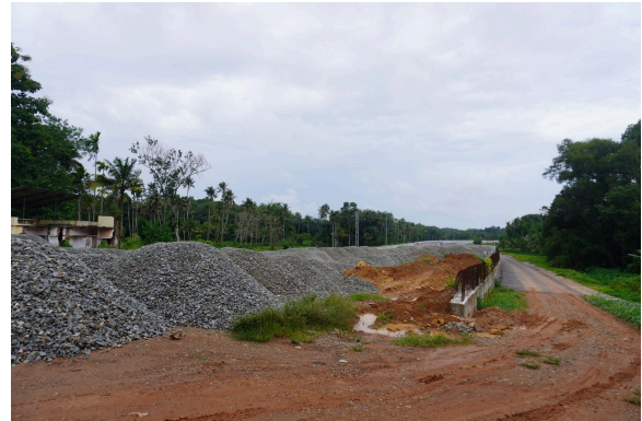
Figure. The new road is being constructed near Keezheveetil kaavu , Kaavu is behind the broken building. Image: P S Soorya, 2024
